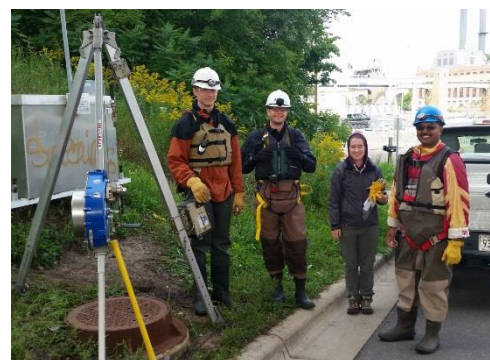
Figure 3. MWMO staff preparing to enter a stormwater tunnel Photograph by B. Faust
